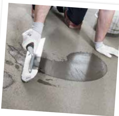
REPAIR LARGE CRACKS
